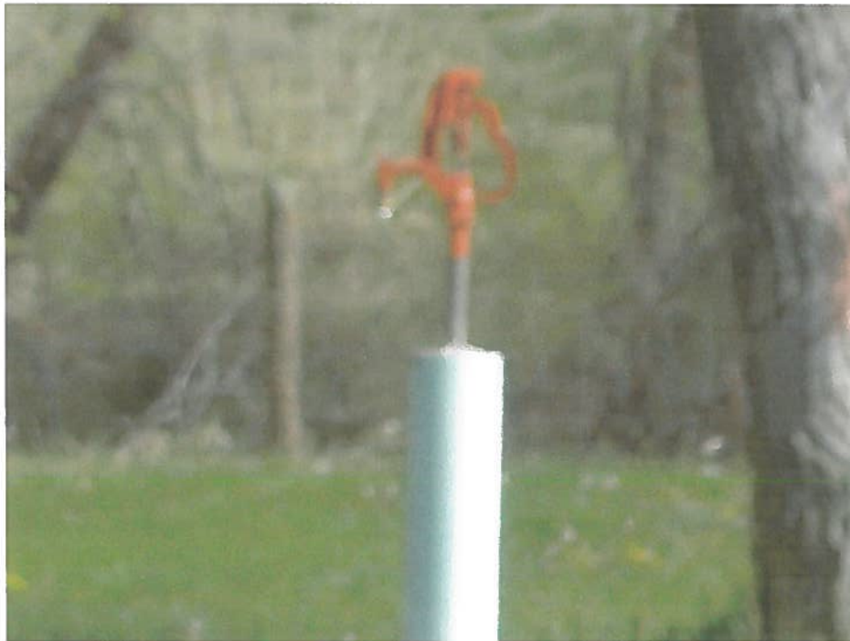
Old Style yard Hydrant
